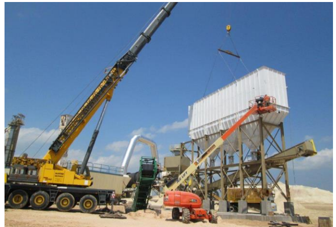
In this sand and gravel facility, a cartridge dust collector replaces an inefficient baghouse to meet EPA emissions standards and improve dust collection efficiency.
