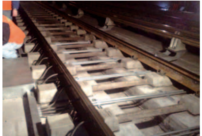
Figure 2: Completely installed and connected measuring eyes
