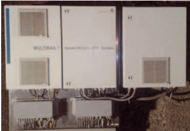
Figure 4: Control electronics in control cabinet form
