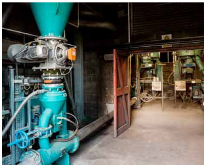
Multicor Feeder for PSP material feeding into the same pipeline as the existing coal feeders
